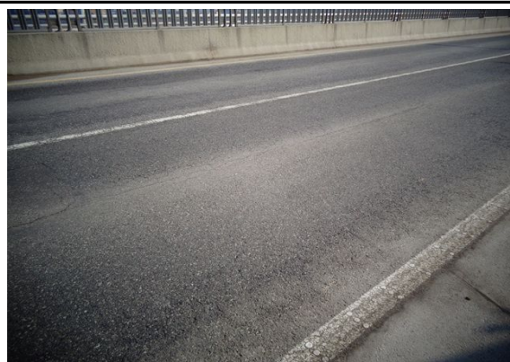
S11 망상균열 (원주방향)
